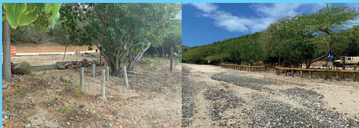
Figure 47: Previously installed and damaged wooden poles (left) have been removed and replaced with new wooden poles and wooden sidewalks (right). (Source: PDC)
