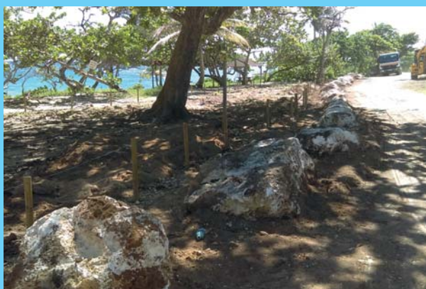
Figure 28: Laying boulders to prevent car traffic on the beach (Source: Adam Gibaud (ONF); 10/22/2020)
